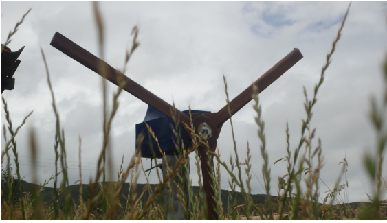
FIG. 11. DIAWIND-A2 wind turbine installed for performance testing in Puntahacienda-Quingeo [7].
